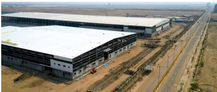
Dholera cell plant (2.5 GW)
