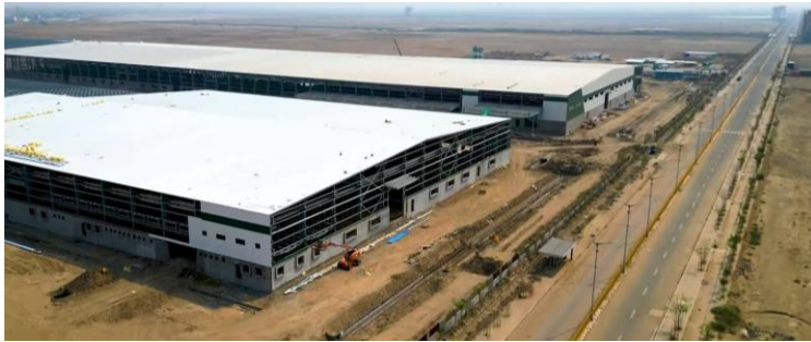
Dholera cell plant (2.5 GW)
